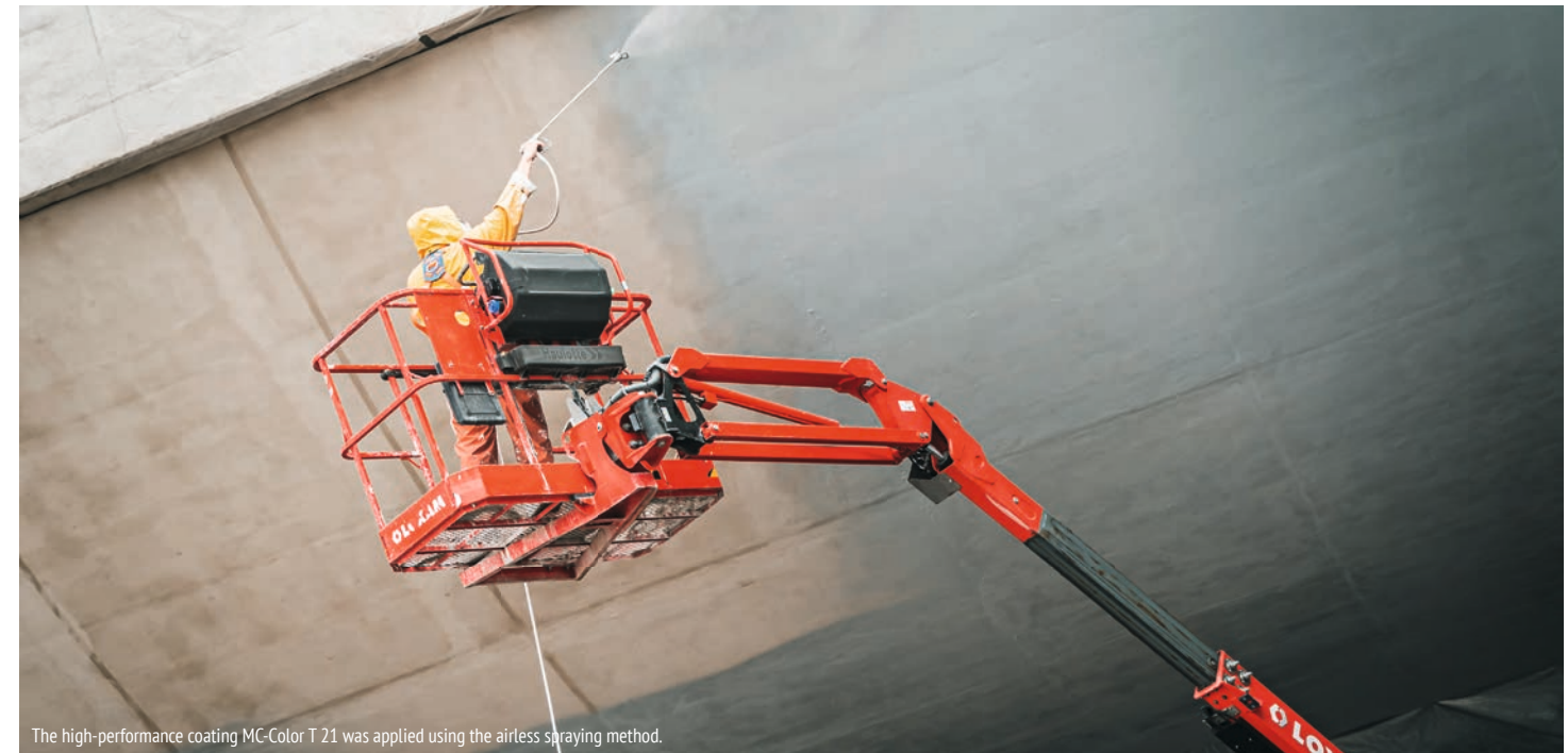
The high-performance coating MC-Color T 21 was applied using the airless spraying method.
