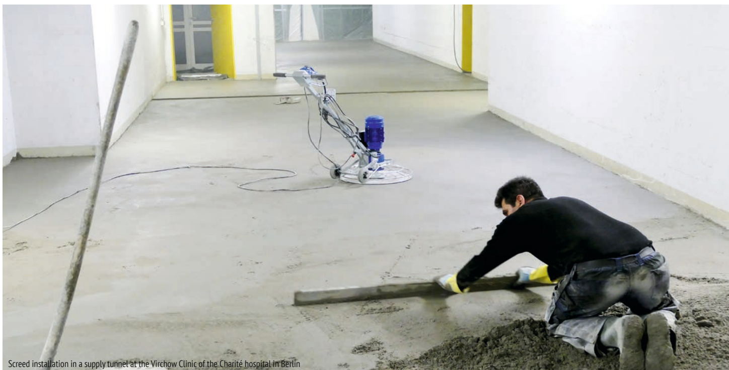
Screed installation in a supply tunnel at the Virchow Clinic of the Charité hospital in Berlin
